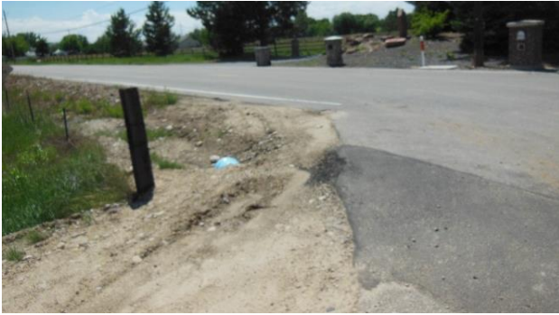
Southeast corner of Bogart Ln and Caswell St (No Sidewalks, Narrow Gravel Shoulder)
