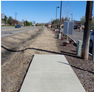
Horseshoe Bend Rd (Example of Incomplete Sidewalks in the Area)
