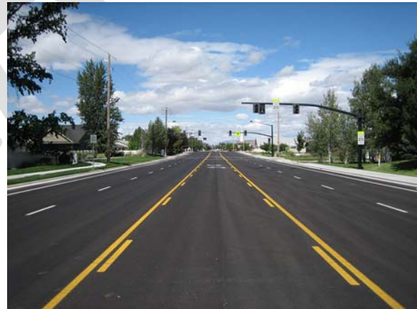
A well-maintained roadway in Meridian. Photo: Shelly Houston, as part of the Your Treasure Valley Future Photo Challenge .
