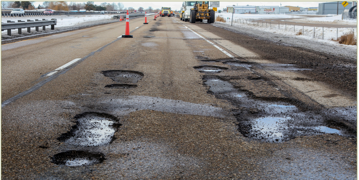
Figure 1. ITD had to advance maintenance work on Interstate 84 to repair huge potholes that resulted from the 2017 winter storms. Photo credit: ITD.
