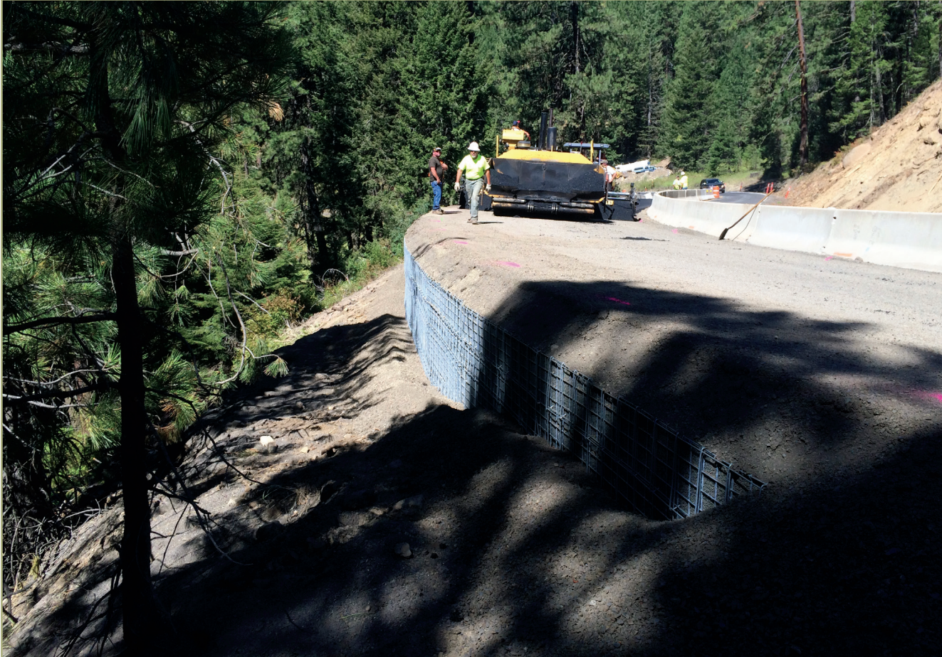
Figure 8. Goose Creek slope stabilization along State Highway 55 near McCall. Photo credit: ITD.
