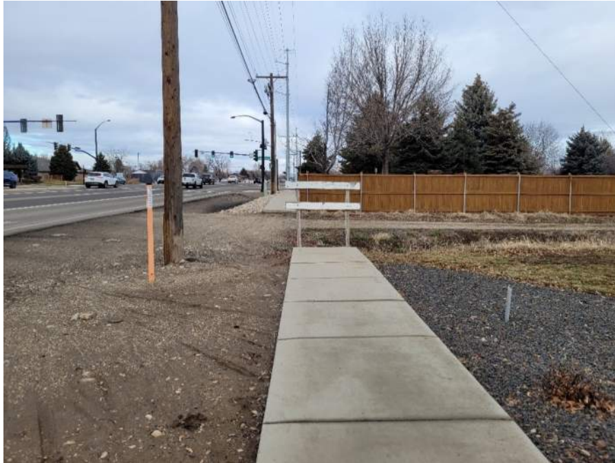
Figure 1-3 | Abrupt shift in sidewalk alignment
