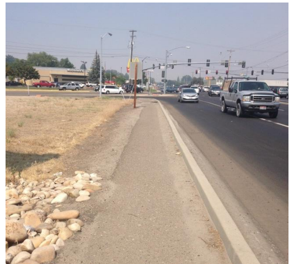
Existing extruded curb walkway on the south side of Chinden Boulevard near Glenwood Street
