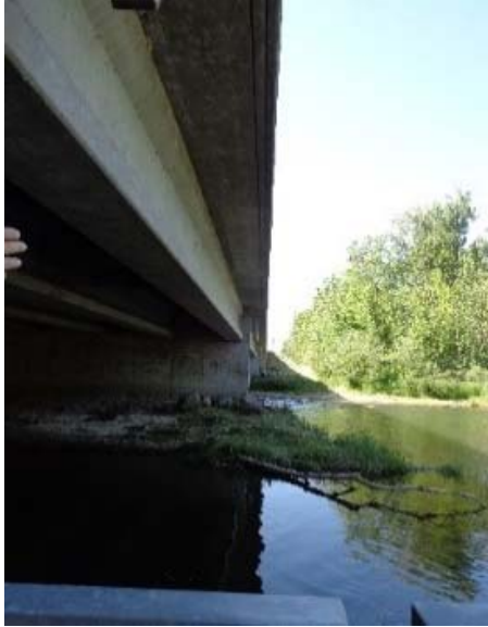
Figure 5: West side of SH-55 bridge, (June 2015) view looking south standing at "Point B" shown on Figure 4, "Bridge Plan View"
