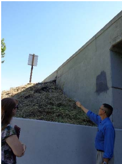
Figure 7: West side of SH-55 bridge, north abutment (June 2015) at northwest corner, "Point B" on Figure 4 - "Bridge Plan View", looking north
