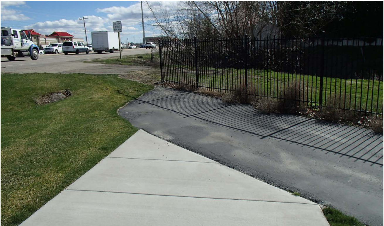
Looking south at the end of existing sidewalk north of South Slough canal
