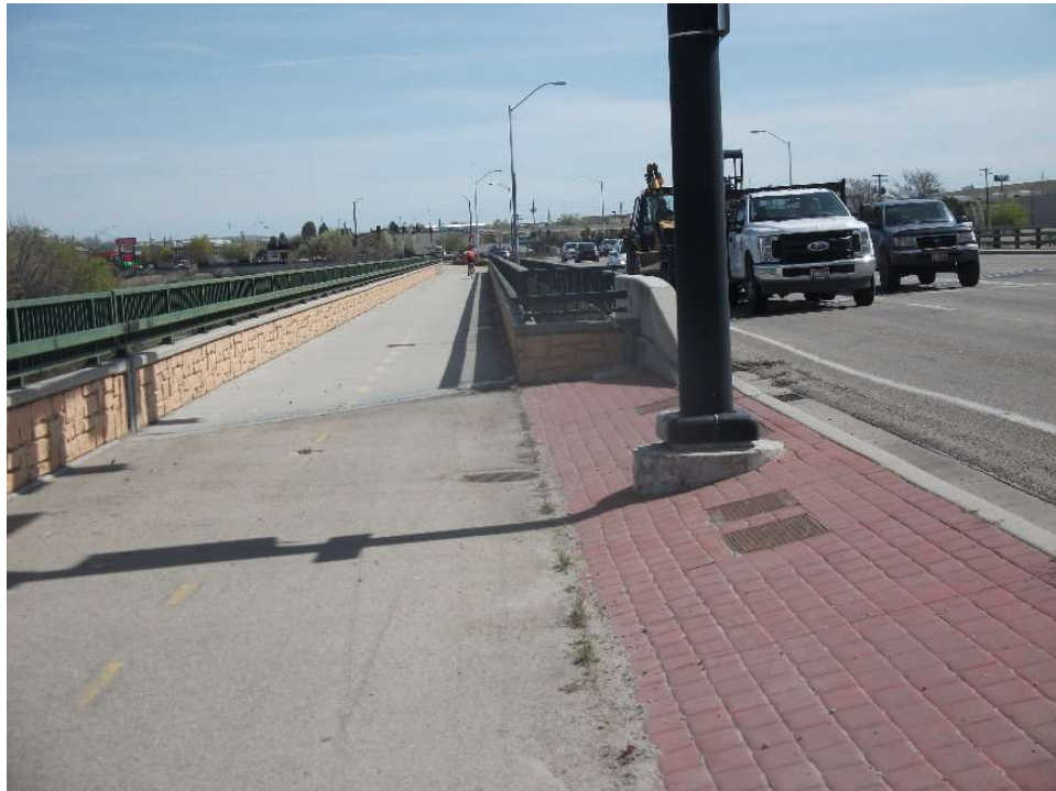
Alternative Route: Southbound Ramp & West Side of Broadway Constraint: Pedestrian Bridge To Cross Gap
