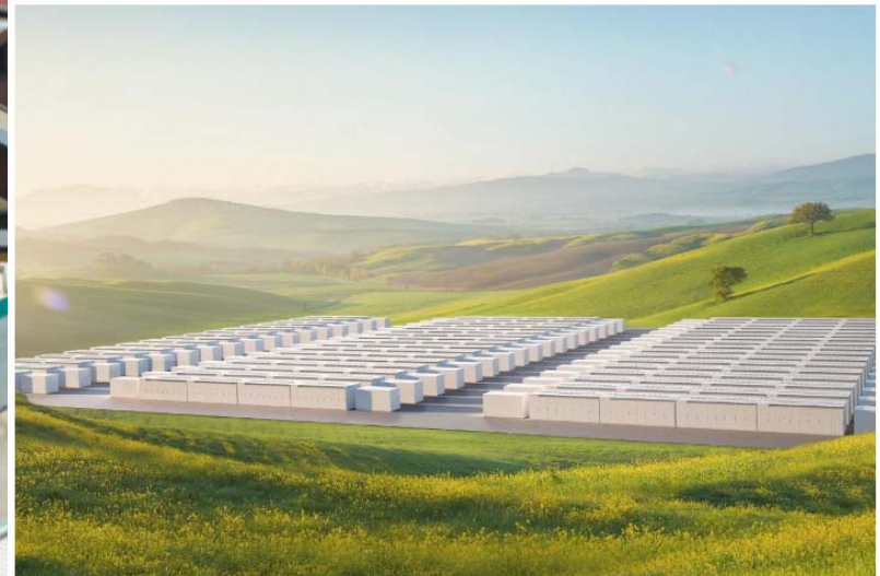
Tesla claims it can deploy an emissions-free 250 MW, 1 GWh power plant in less than three months
