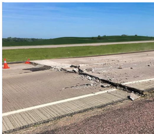
Figure 4: Pavement Buckles in Vermillion, South Dakota (2019). Source: South Dakota Highway Patrol
