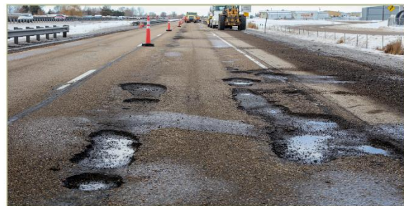
Figure 6: Potholes on I-84 resulting from the 2017 winter storms, Source: ITD, COMPASS
