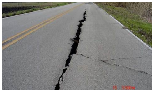
Figure 3: Drought-Related Severe Pavement Crack in Travis County, TX (2005). Source: CAMPO
