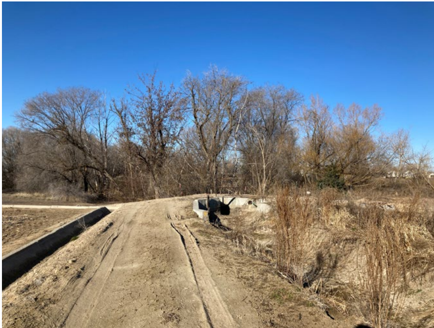
Foothill Ditch, looking west toward Alternative A ditch crossing: culvert extension and security fencing needed
