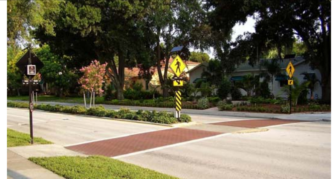
IA-21 3.a For any approach two RRFB required, One on right-hand and one on left-hand of roadway. If divided highway left-hand should be installed on median if practical rather than far left-hand
